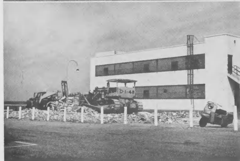
RAZED IN June was the concrete-block Field Engineering Office which was located east of the General Office Building. The 1000-square-foot structure was erected in 1941. NA JUNI a worde tumbá e oficina di concreto di Field Engineering cu tabata situá net pariba di Oficina Mayor.
